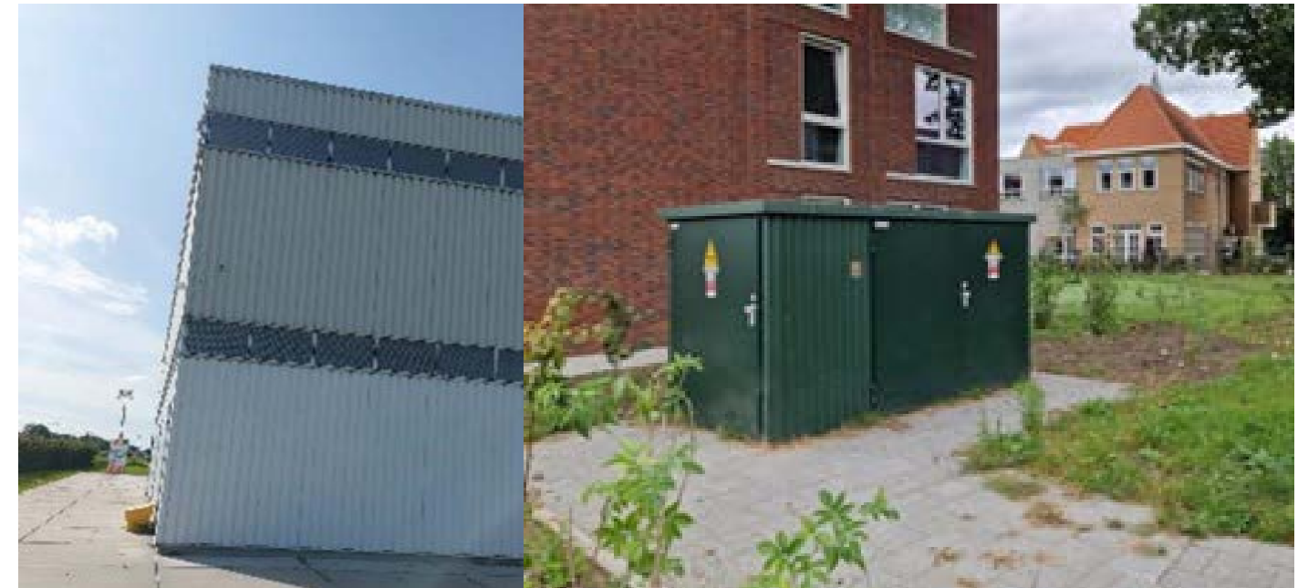
Hoogspanningsstations (onderstation) | Midden-laagspanningstation (MS/LS)
